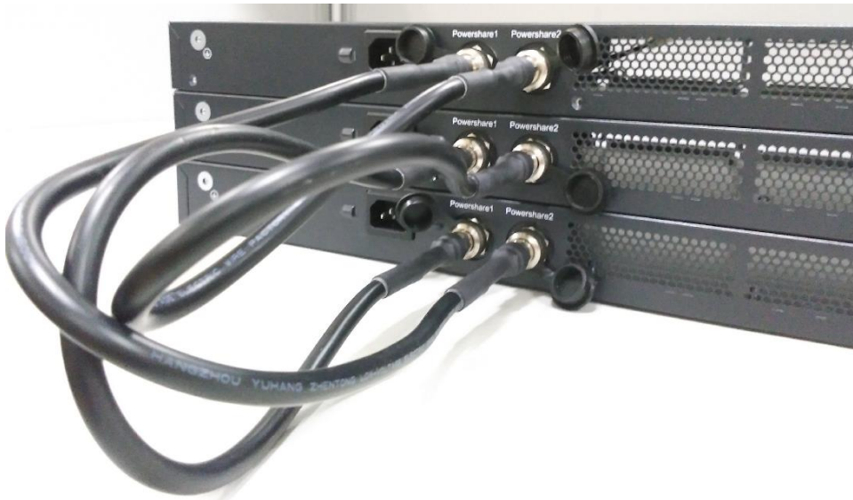
Figure 3-12 Connecting Cables Among Three Switches 3
