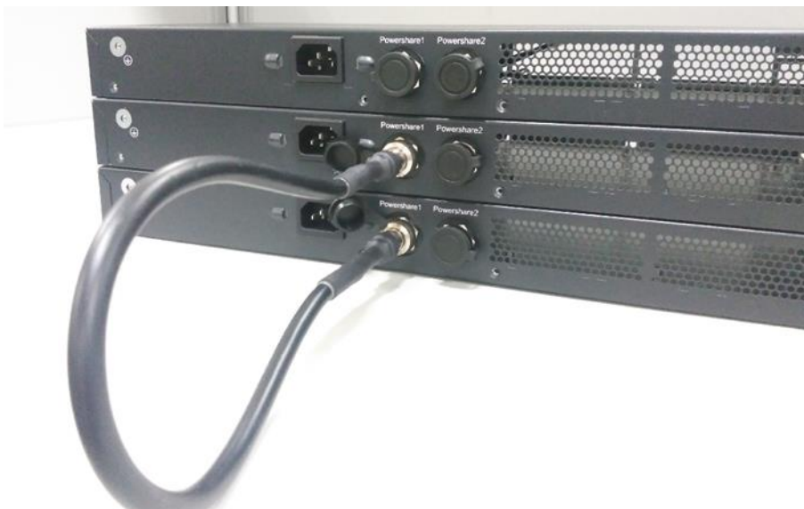
Figure 3-11 Connecting Cables Among Three Switches 2
