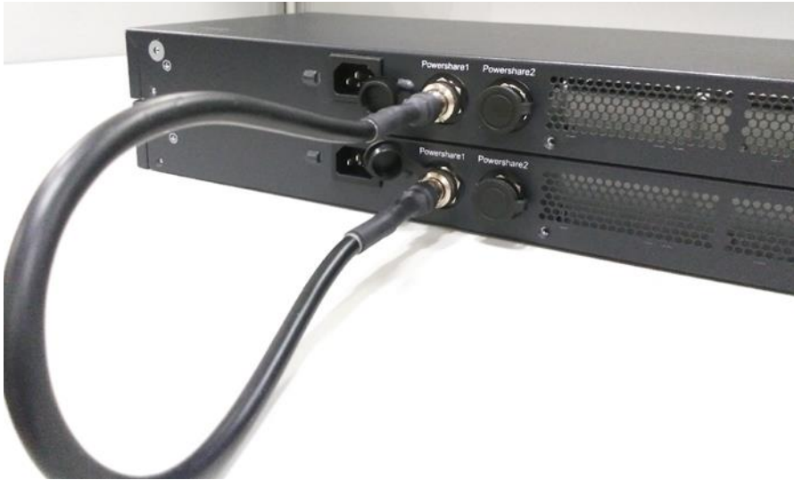
Figure 3-9 Connecting Cables between Two Switches
